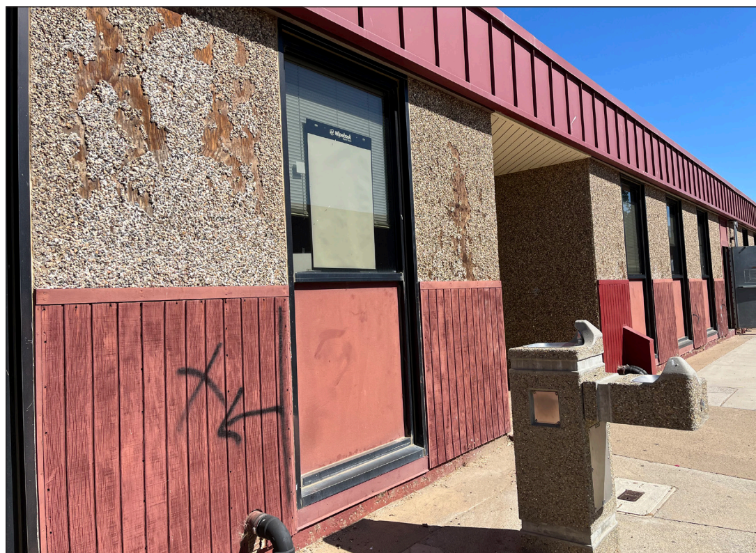
The outer layer of Mountain Empire High School's walls has been peeled away by the wind. These walls are supposed to be the school's defense against wind, fire and earthquakes.
